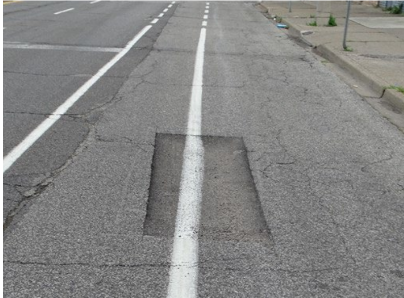
Figure 8: Pavement Depression near 1451 University Avenue
