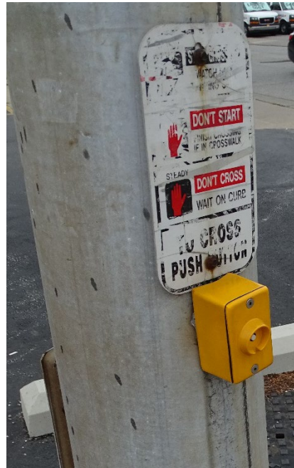
Figure 3: Non-AODA Compliant Pedestrian Push Button
