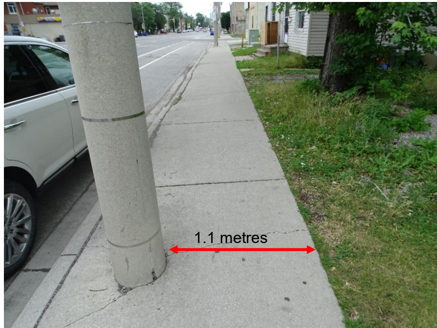
Figure 2: Sidewalk Width Reduced by Hydro Pole
