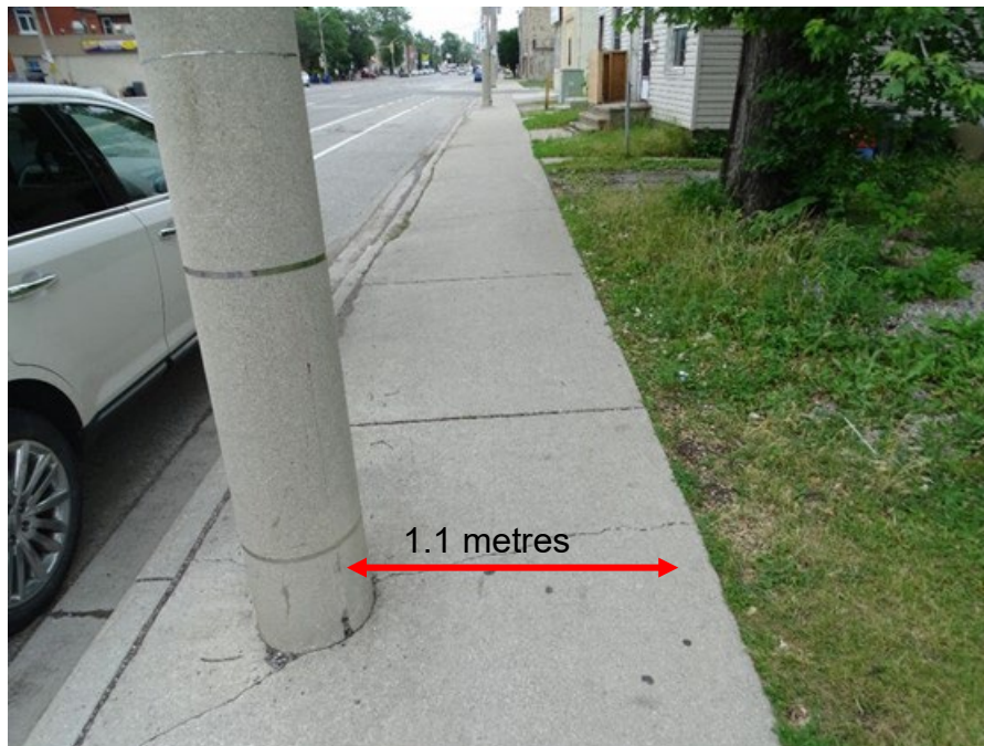
Figure 12: Sidewalk Width Reduced by Hydro Pole
